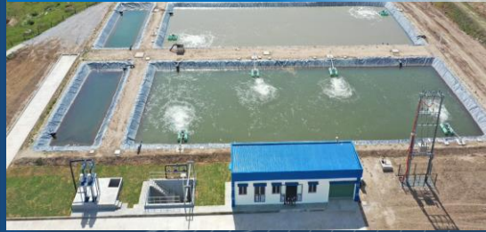
Biological Waste-Water Treatment
